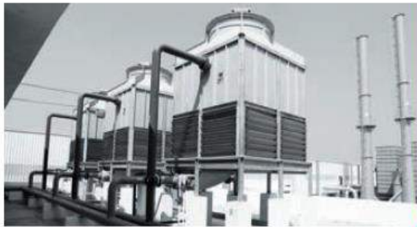
Chilling plant cooling towers New plant at Hunegundipalle village
